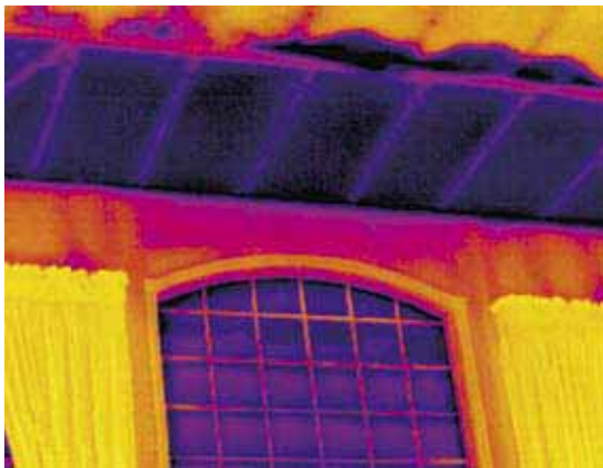
This thermographic image shows missing insulation and demonstrates a diagnostic tool used by MaGrann Associates.
